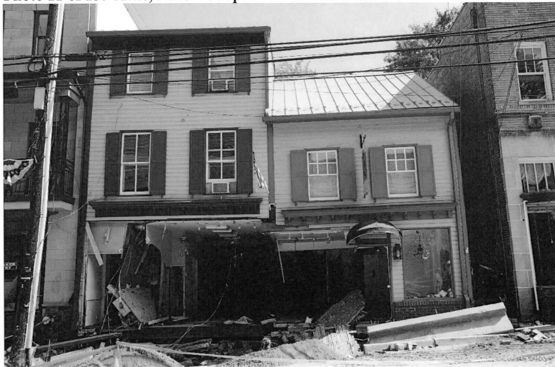
Photo 12 of 13: North elevation, 8109 & 8113 Main Street following 2016 flood. 08/02/2016
