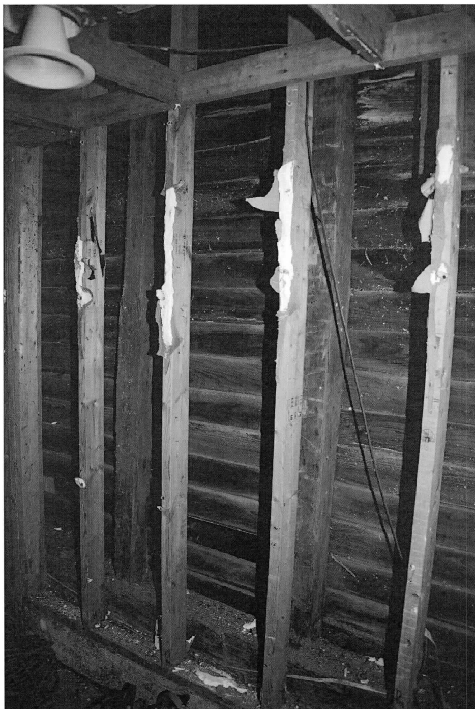
Photo 13 of 13: 8113 Main St., first story north wall framing following 2016 flood, prior to removal. 3/22/2017
